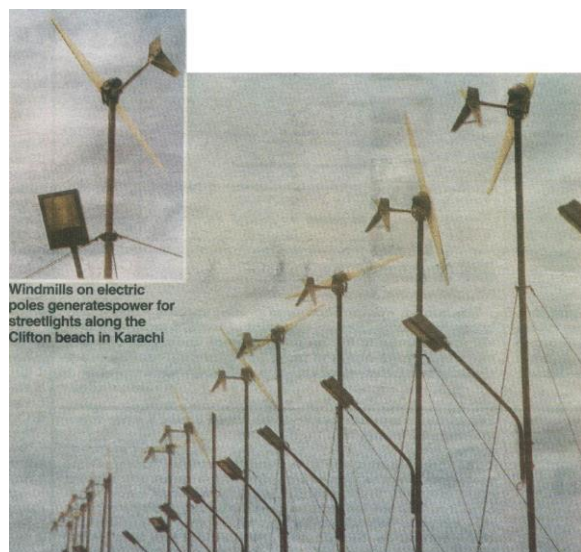
Figure 1: So-called wind farm installed at Karachi Beach and failed after few weeks.
